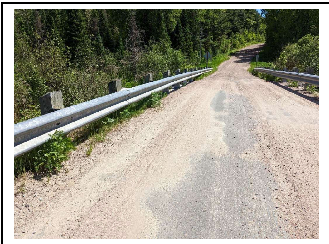
Photo 8 Longitudinal grooves on structure wearing surface
