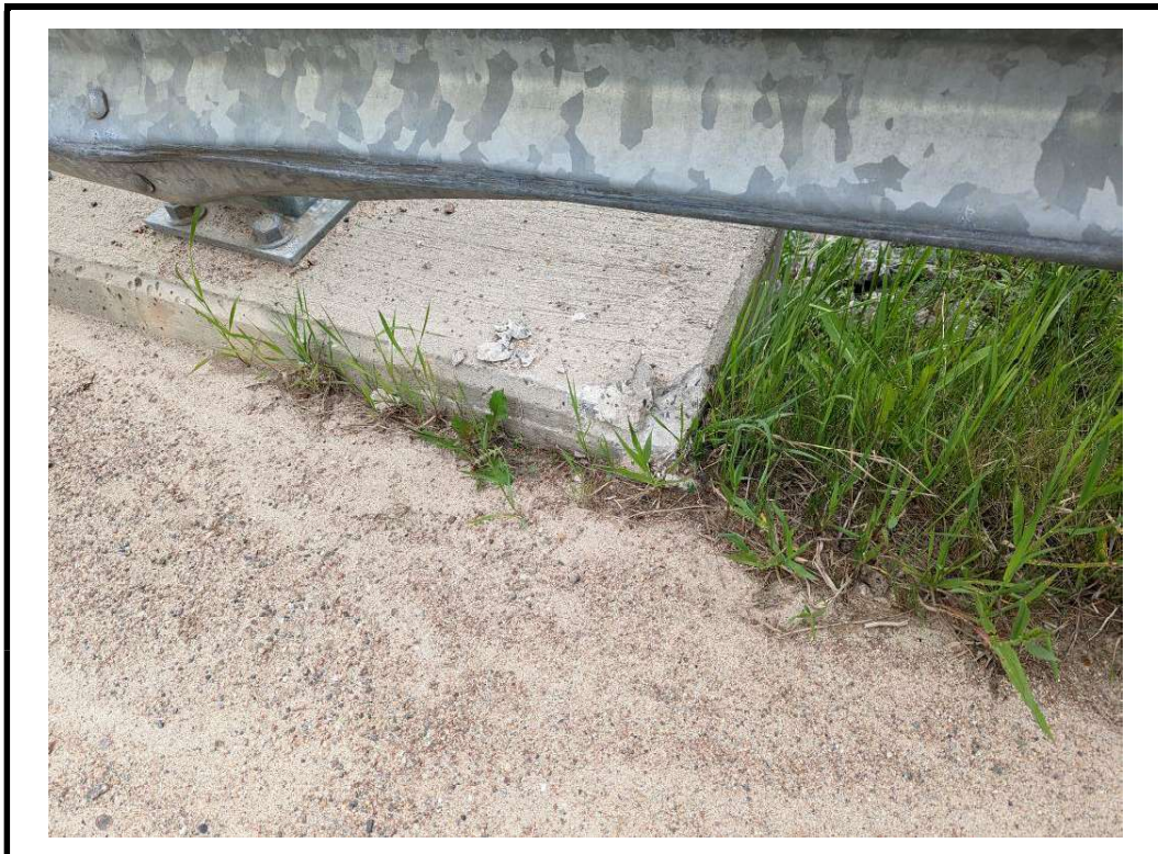
Photo 12 Small spall noted in curb at southeast corner
