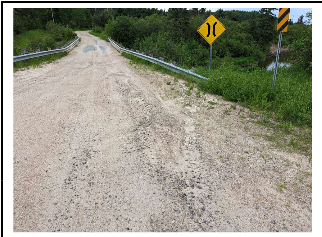
Photo 10 Washout noted in wearing surface at north approach
