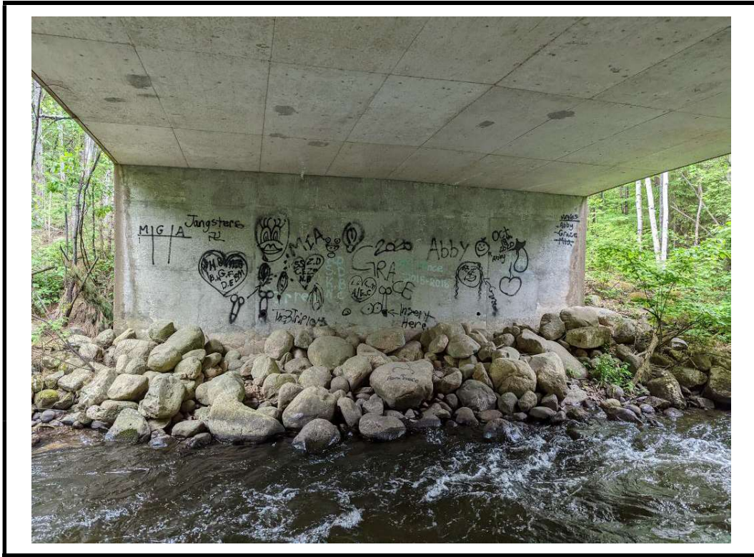
Photo 13 Graffiti on south abutment wall
