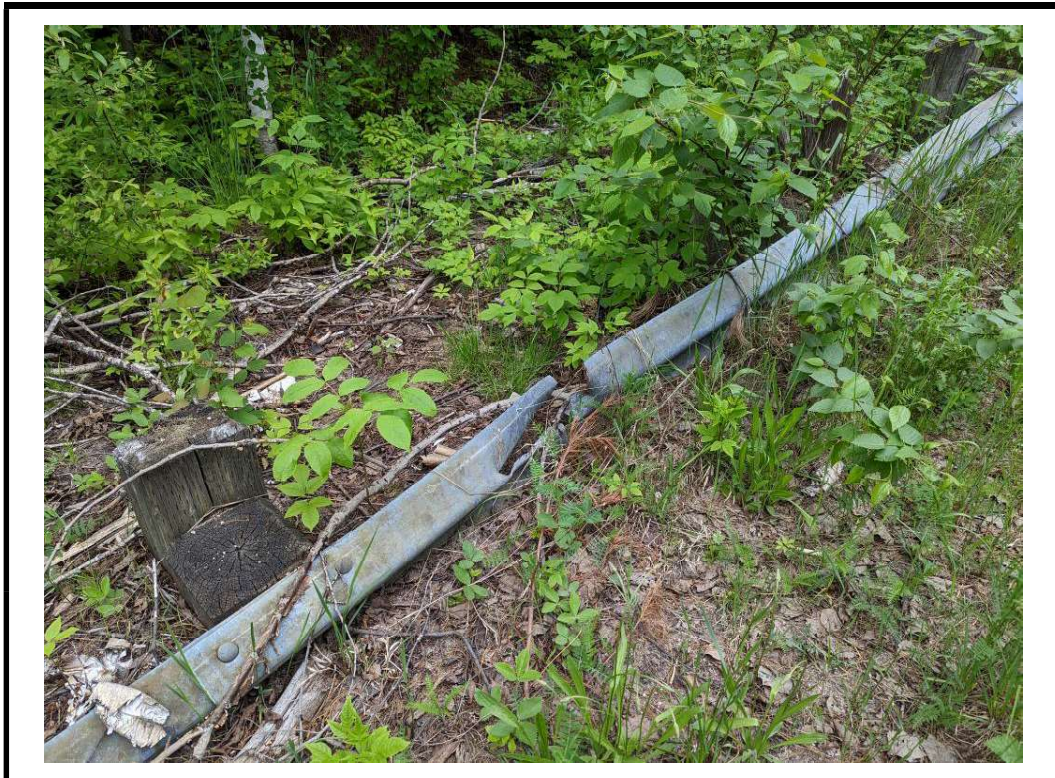
Photo 8 Damage observed on steel beam at southwest corner
