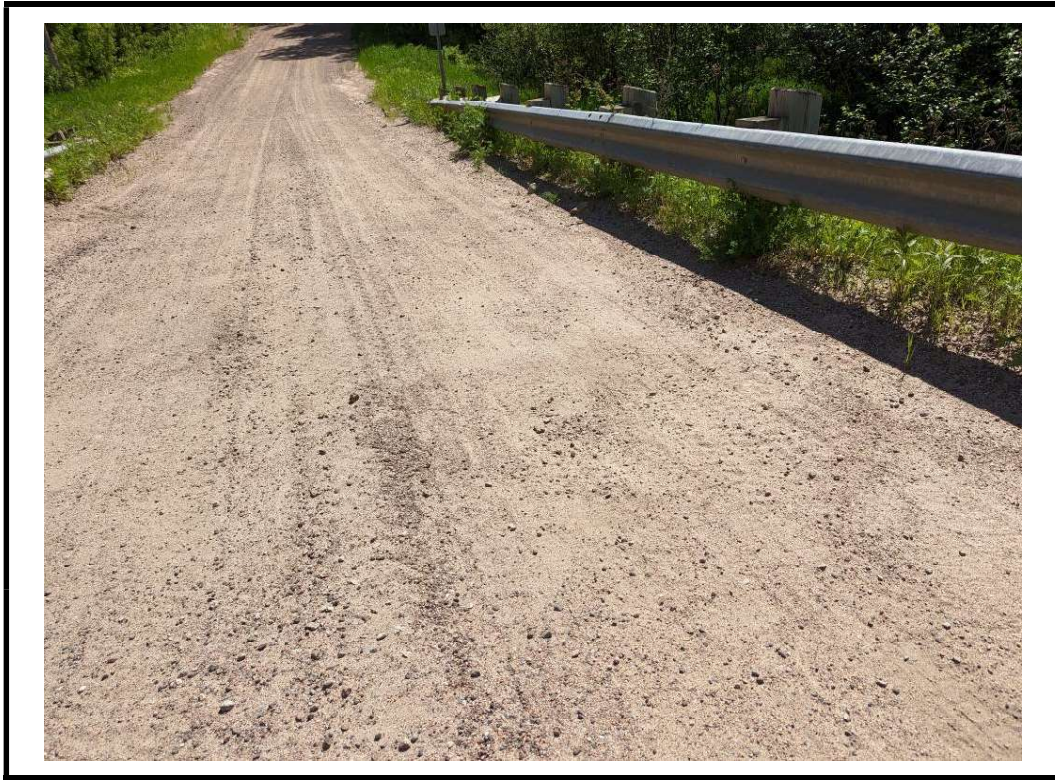
Photo 7 Tire rutting and loose gravel on east approach.
