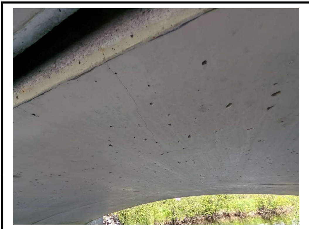
Photo 10 Narrow transverse crack noted in centre of soffit at south end
