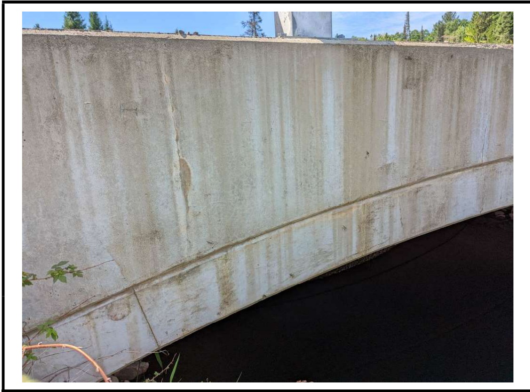
Photo 9 Stained map cracks noted on exterior face of soffit
