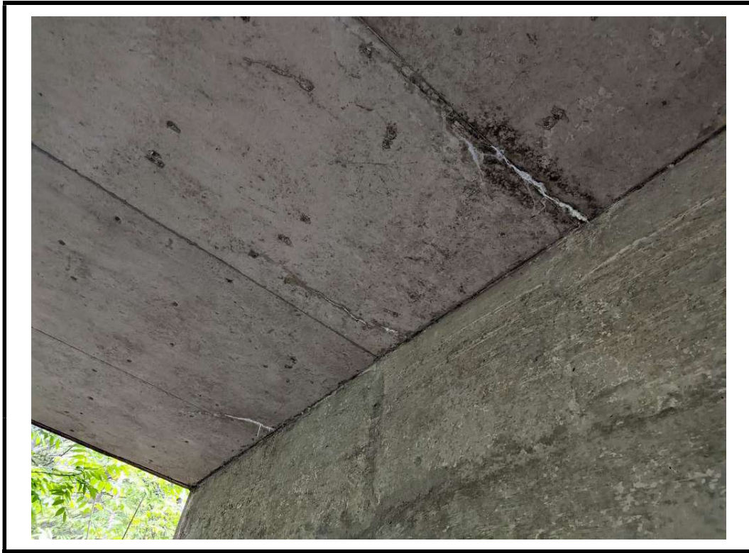
Photo 9 Narrow crack with efflorescence on north deck soffit
