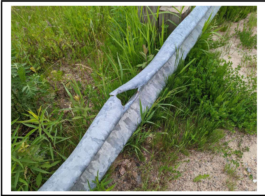
Photo 7 Collision damage noted on approach barrier at northeast corner
