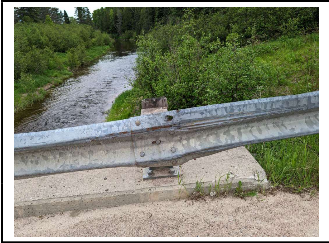
Photo 9 Vehicle damaged noted on deck barrier at southeast corner
