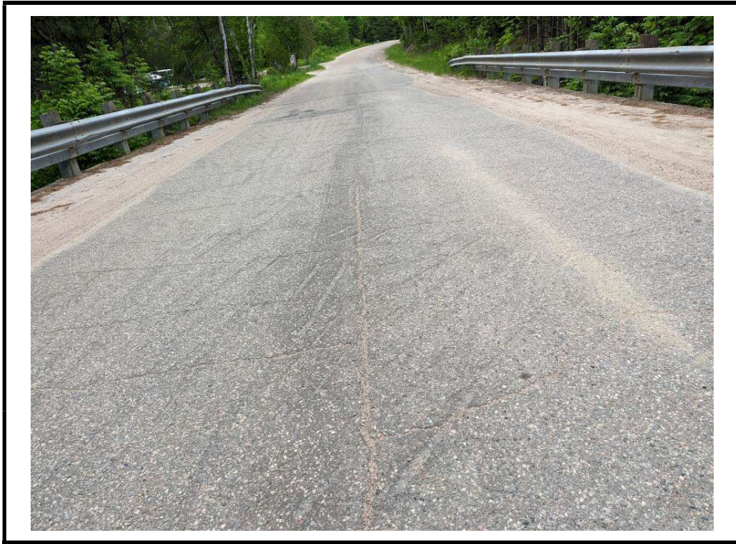
Photo 7 Wide longitudinal and transverse cracks noted on wearing surface
