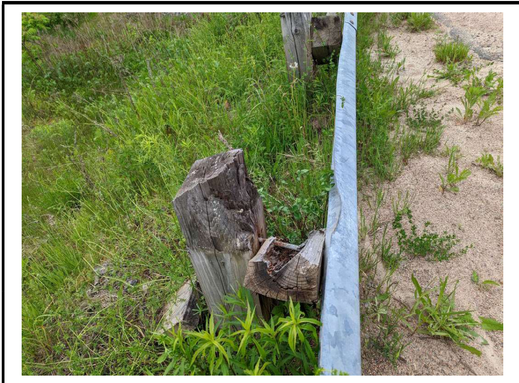
Photo 8 Checks and splits on barrier post with damaged and rotated spacer block
