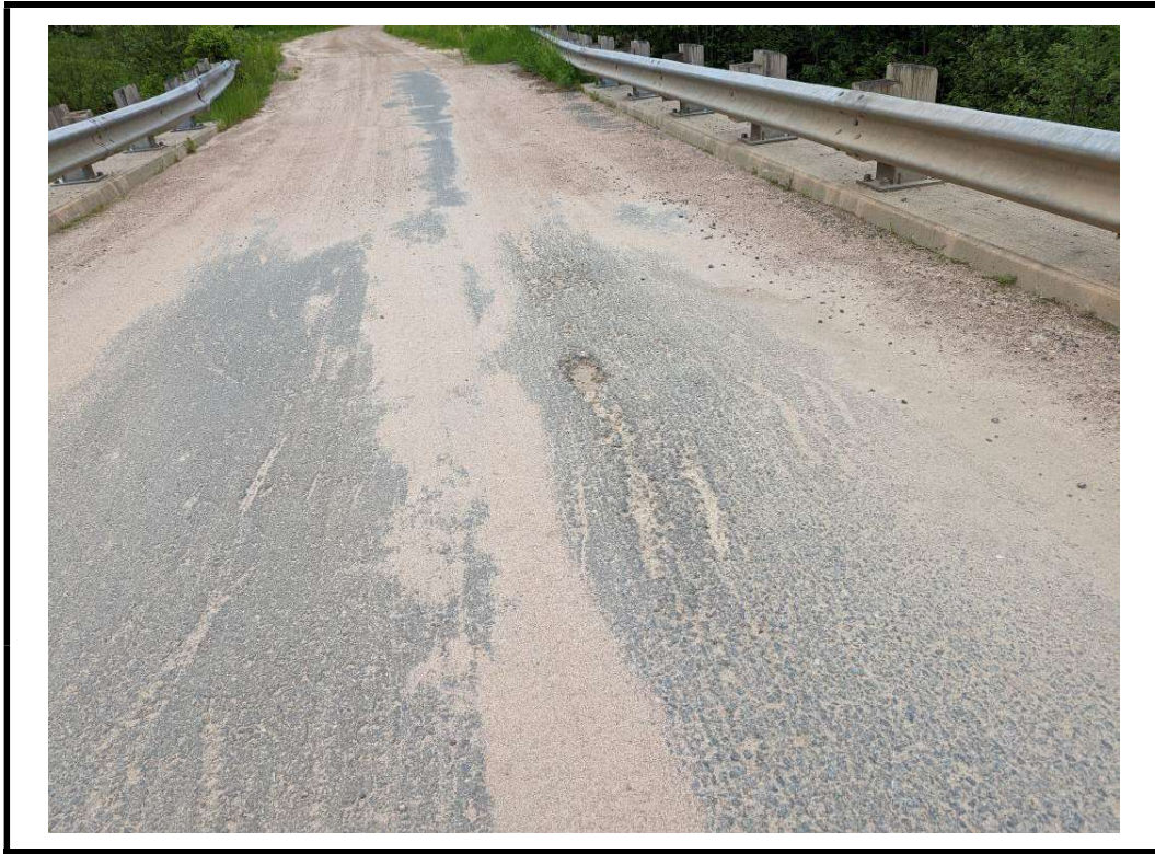
Photo 11 Minor scaling and small gouges noted in middle of deck wearing surface
