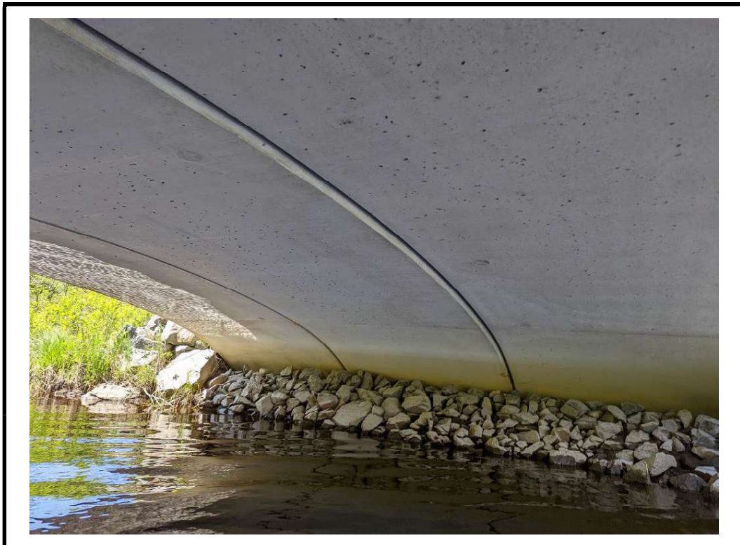
Photo 12 Bug holes noted throughout barrel soffit
